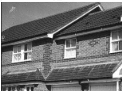
Roof tiles spoiled by run-off staining.
